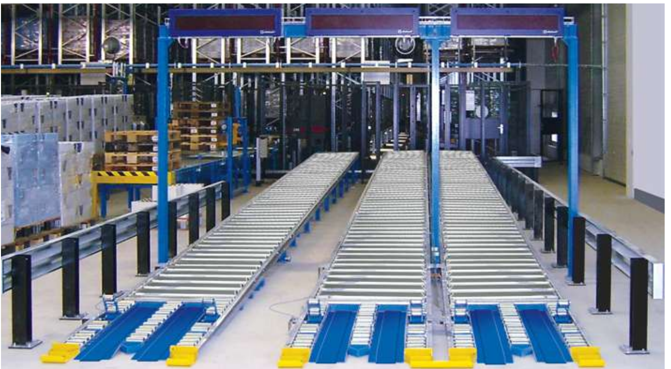
Shipping track with reinforced removal station
