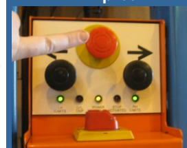
Push button controls
