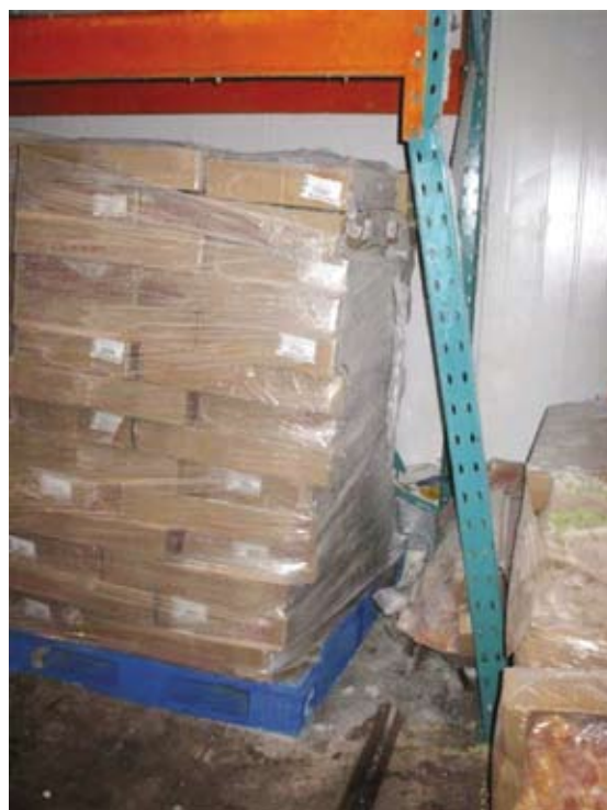
Racking damage in a cold store
