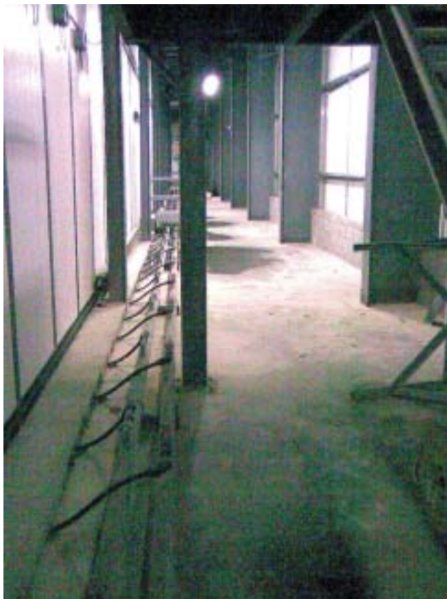
Glycol underfloor heating installation showing the main supply and return pipes and the plastic pipes that go under the cold room floor.
