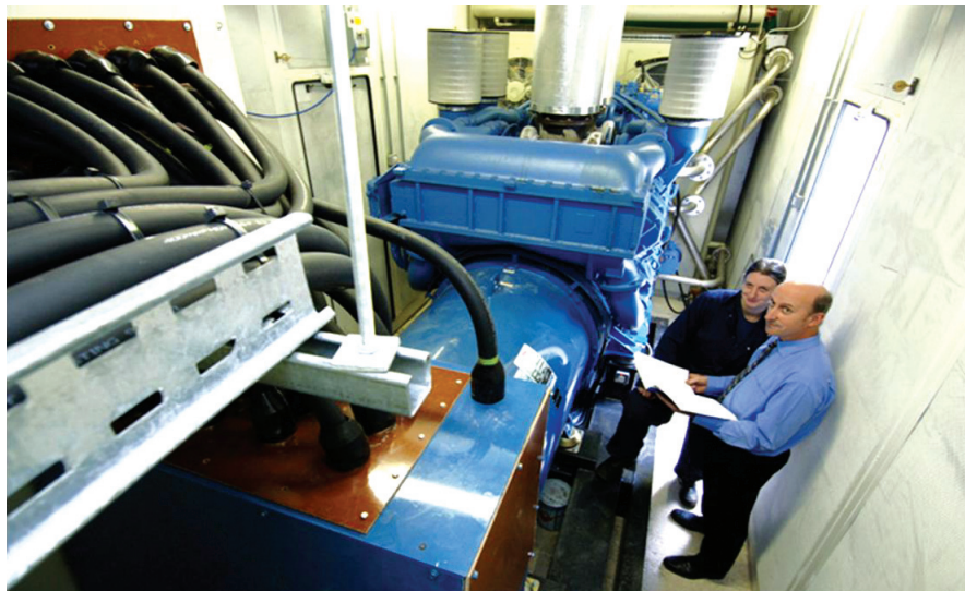
One of the generators at Reed Boardall.
